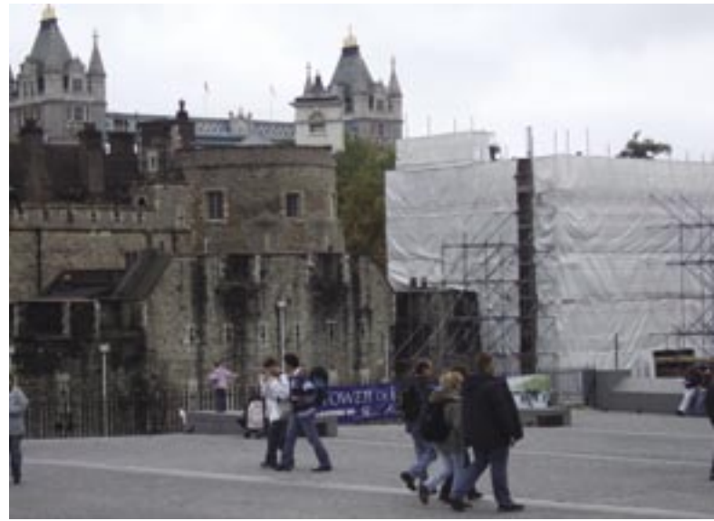
The Tower of London (with Tower Bridge in the background) undergoing essential repairwork.
