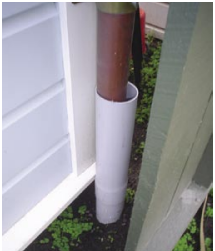
The finished product, a copper downpipe with a PVC sleeve on a new building, circa 2006.
