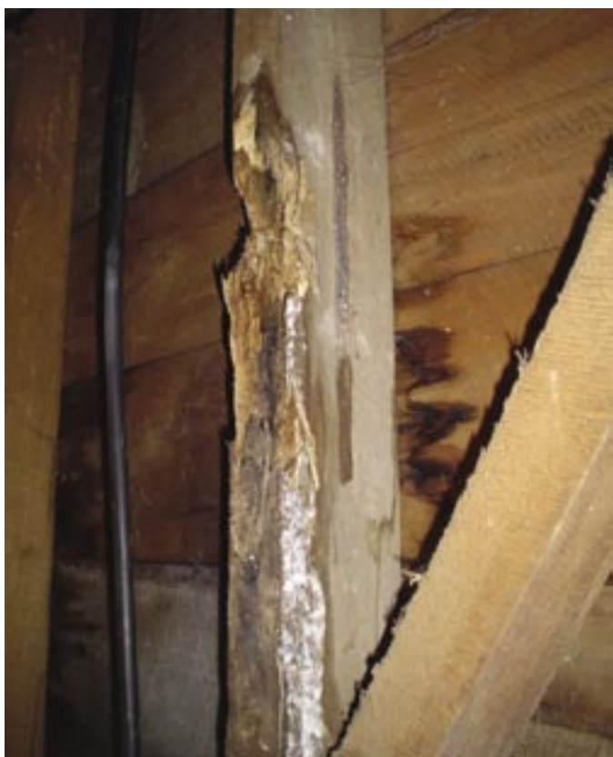
Timber that has rotted due to leaks in a polybutylene piping joint, uncovered when an infinity system was being installed and the piping ruptured.
