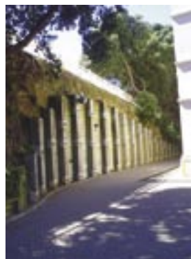
What might have been... Straight Up-and built-to-last (but taxpayer funded) – a retaining wall opposite the General Assembly Building, Parliament Grounds, Wellington.
