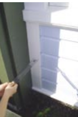
Straight and narrow...Ruler shows width of boundary gap, house built 2006.
