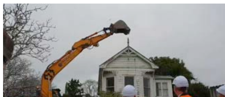
Demolition has started in Onehunga to make way for 42 apartments - 25 of which will be KiwiBuild.
