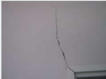
A further example of sheet breakage requiring replacement
