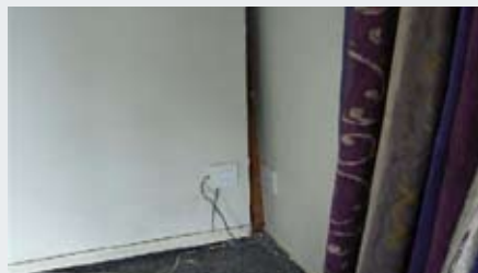
Lining detached from the framing requiring replacement of the bracing element
