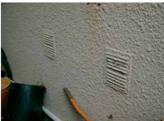
Example of Blocked Ventilation Vents
