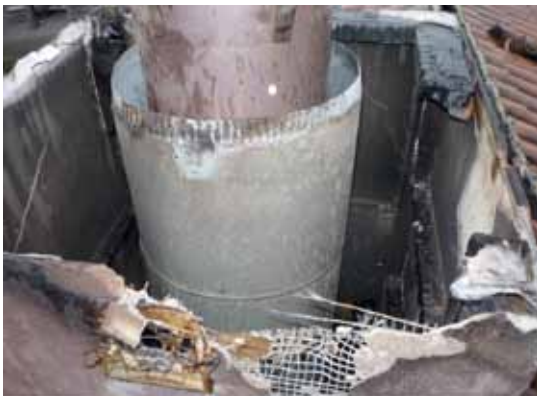
Fire Damage from a Built-in Woodburning Appliance.
