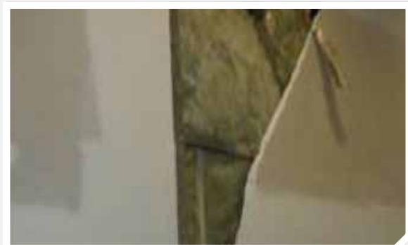
Figure 1: Substantial damage to non-structural gypsum plasterboard partition
