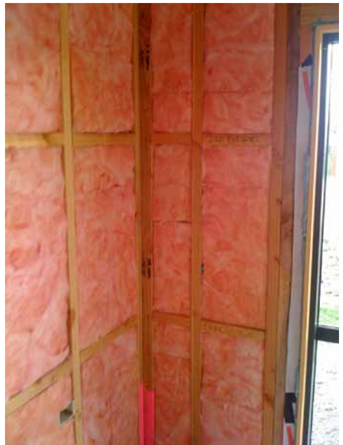
Good installation in the Havelock North Best Home – tightly fitting with no tucks or folds.
