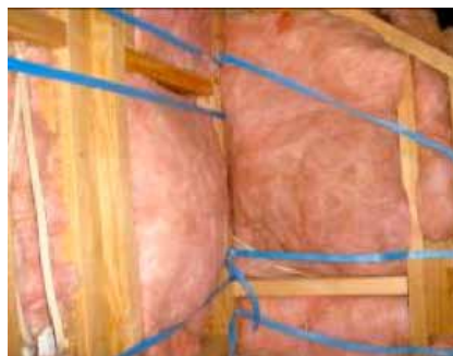
Compressed and slumping insulation – it needs to be a good even fit to work effectively.
