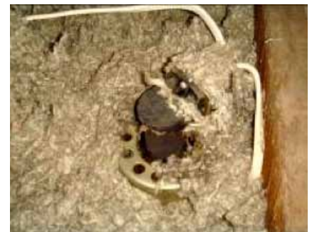
Loose fill has covered this downlight – this is a significant fire risk.
